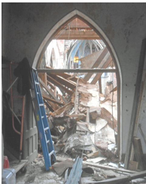
Transfiguration Church roof collapse
